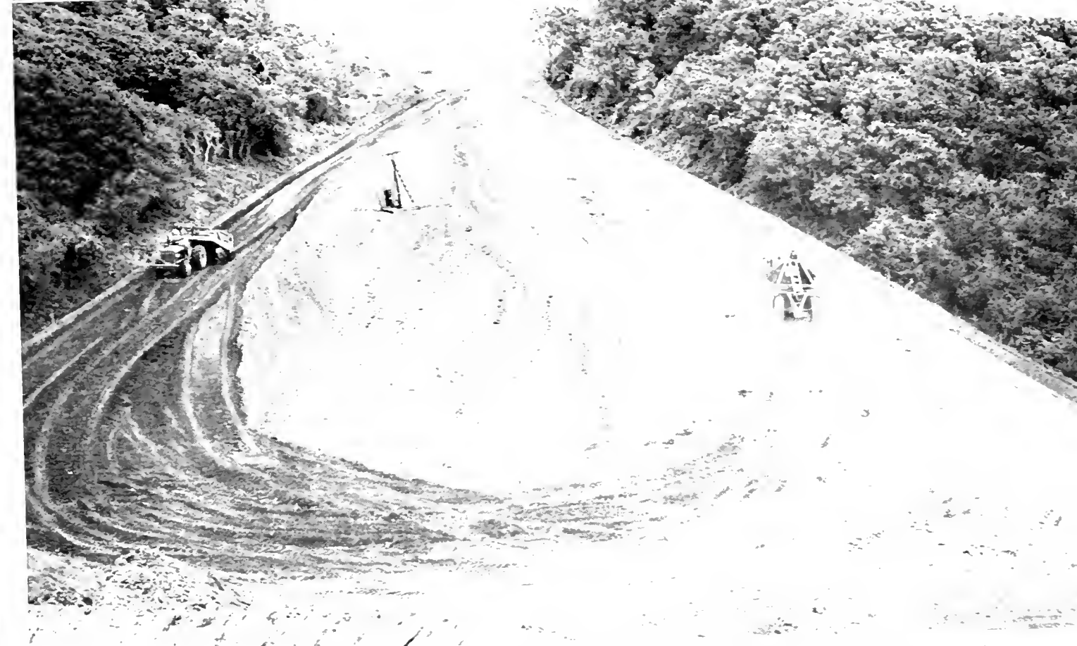
Construction on new Red Key-Watson, e Highway, is proceeding rapidly. Upper—Truck loading with tractor pushing. In right foreground, Bulldozer in operation and in background, two Turnabouts hauling to fill. Lower—Huge fill being made.
